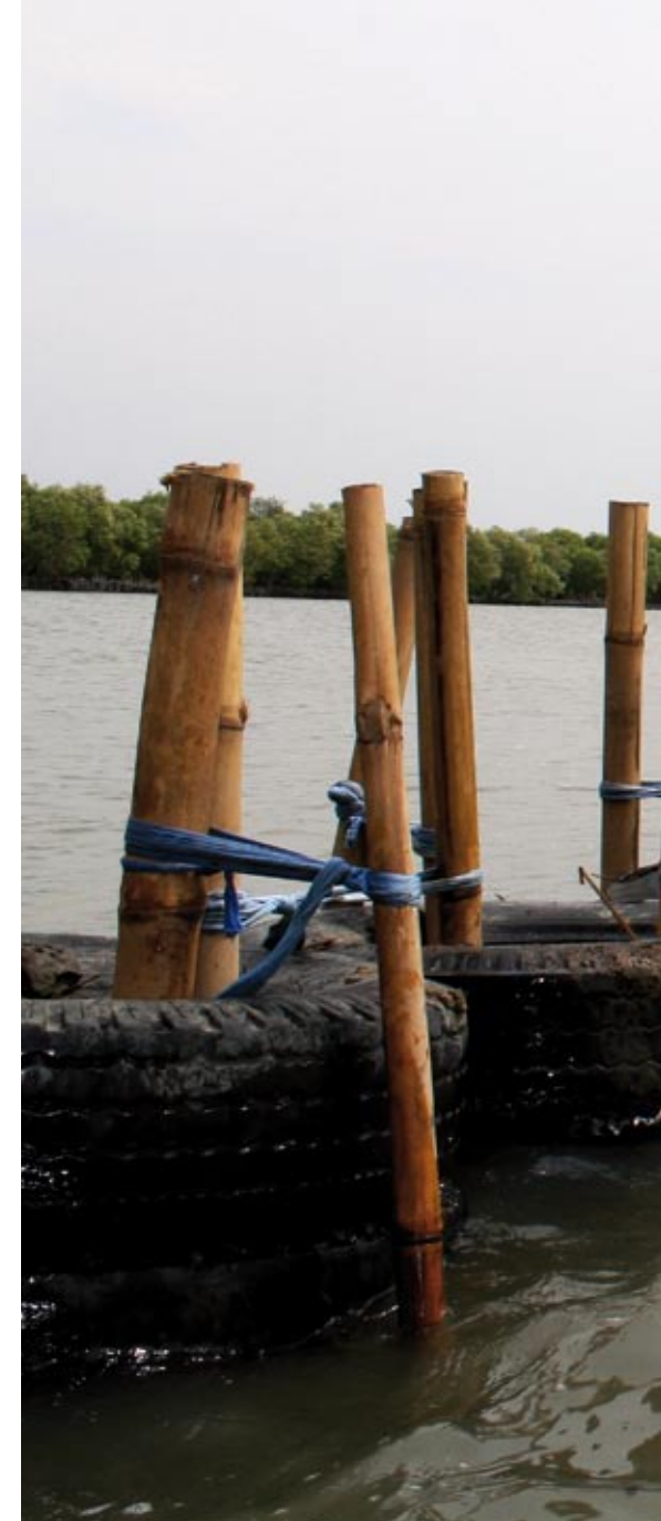
01 - Breakwater device made of used tyres, Tugurejo sub-district
